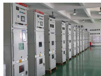
High voltage soft start cabinet
