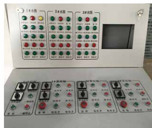
Centralized control console
